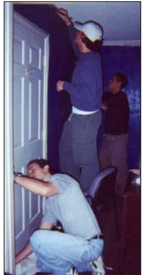
LULAC scholarship recipients paint the Tennessee State Office in preparation for its opening.
